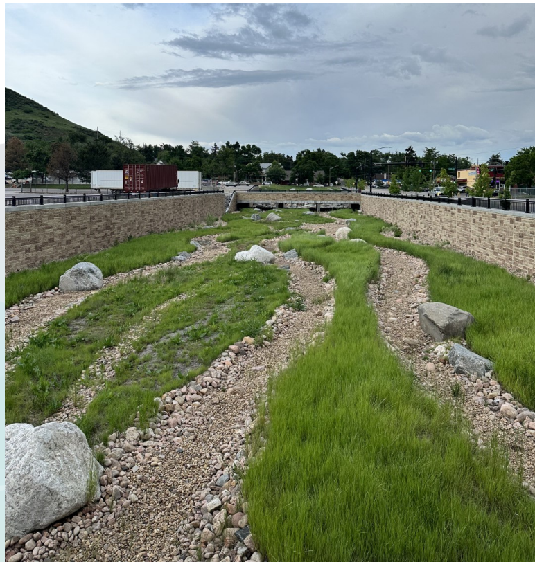
This former concrete box culvert has been transformed into an open channel, native soil, vegetated greenway
