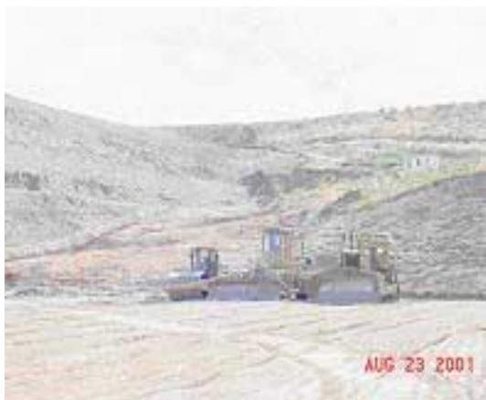
HORSETOOTH DAM – The north dam at Horsetooth Reservoir is being reconstructed in two major phases.
