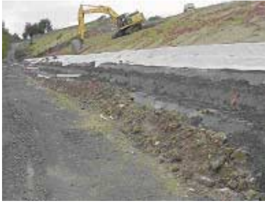
LEYDEN DAM -- During the tour, CASFM members watched granular bedding being placed on the embankment.
