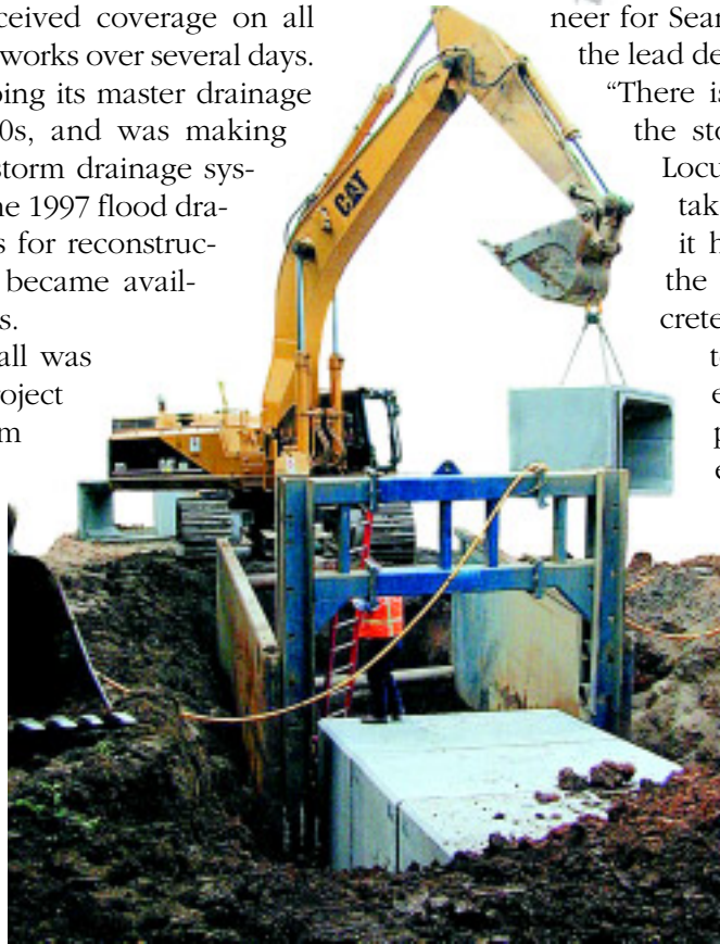
The trench box used during installation of 8-ft. x 5-ft. reinforced concrete box sections allowed for smaller excavation and minimized site problems from wet weather runoff.
